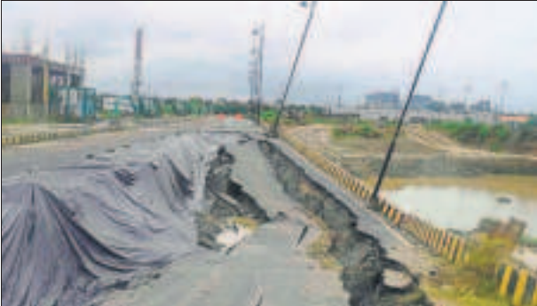
A large stretch of road caved in near Ekana Stadium DEEPAK GUPTA/HT
